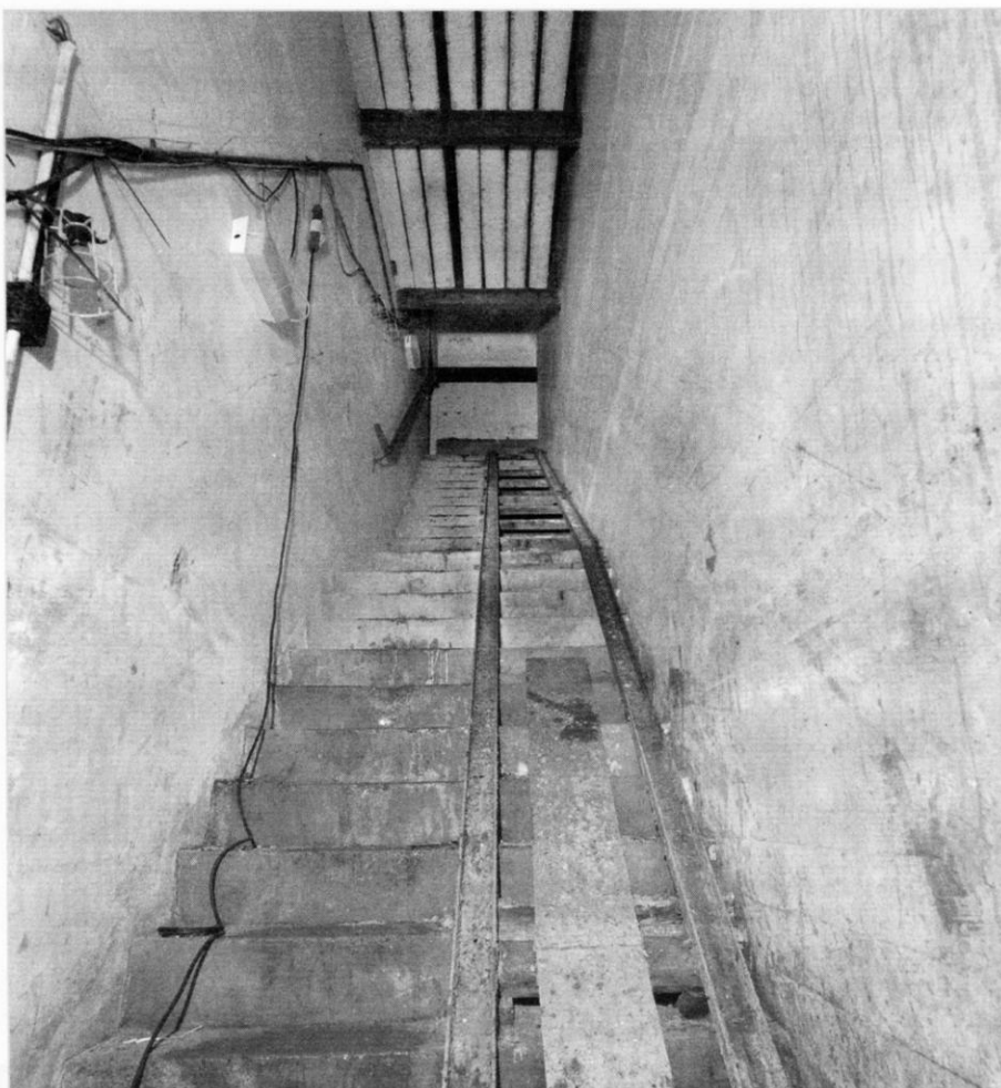
The west stairs between the basement and sub-basement. Note the rails for moving a wheeled cart between floors. Photo by Nick Catford
